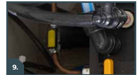
9. GAS ISOLATION VALVE
