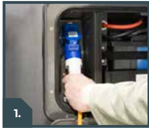
1. POWER SUPPLY TO OPUS
