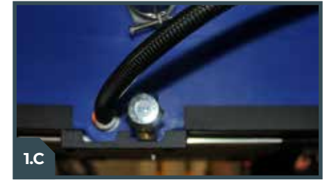
1.C WATER TANK TAP
