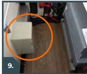
9. LOCATION OF CIRCUIT BREAKERS
